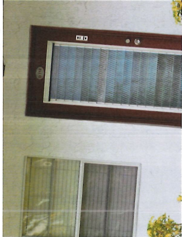
Unprotected Glazed Entry Door
