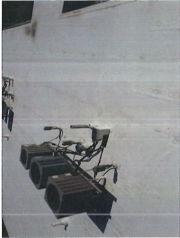
Membrane Roof Covering
